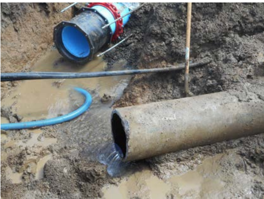
2688- West End – Severed Transite waterline
